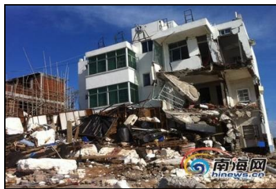
Figure 34. The hazards of Rammasun in Wenchang, Hainan
